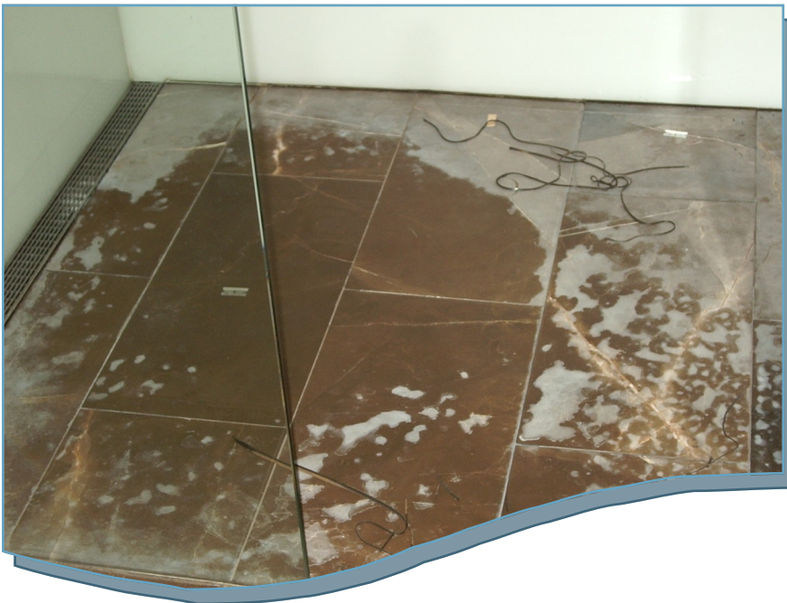
Example of efflorescence
